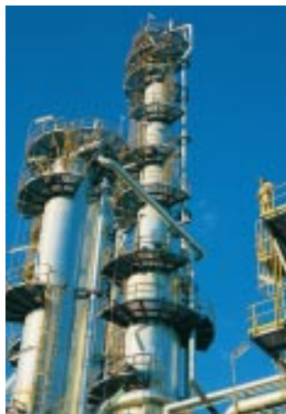
Right Duty site controller, Marten Noordzy, on a platform at the newly commissioned ammonia plant at Kwinana in Western Australia.
